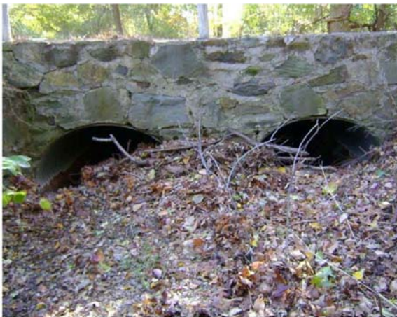
Photo source: CRC; Yard waste blocking a culvert
