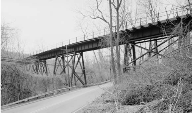
Above: Library of Congress Photo of the trestle bridge over Route 29 (State Road) currently owned by Norfolk Southern and would be made part of the Devault Trail.
